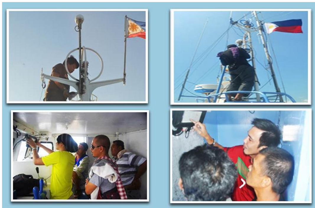
Fig. 1. Installation and trial operation of MARLIN onboard catcher vessel including VMS MTU.
