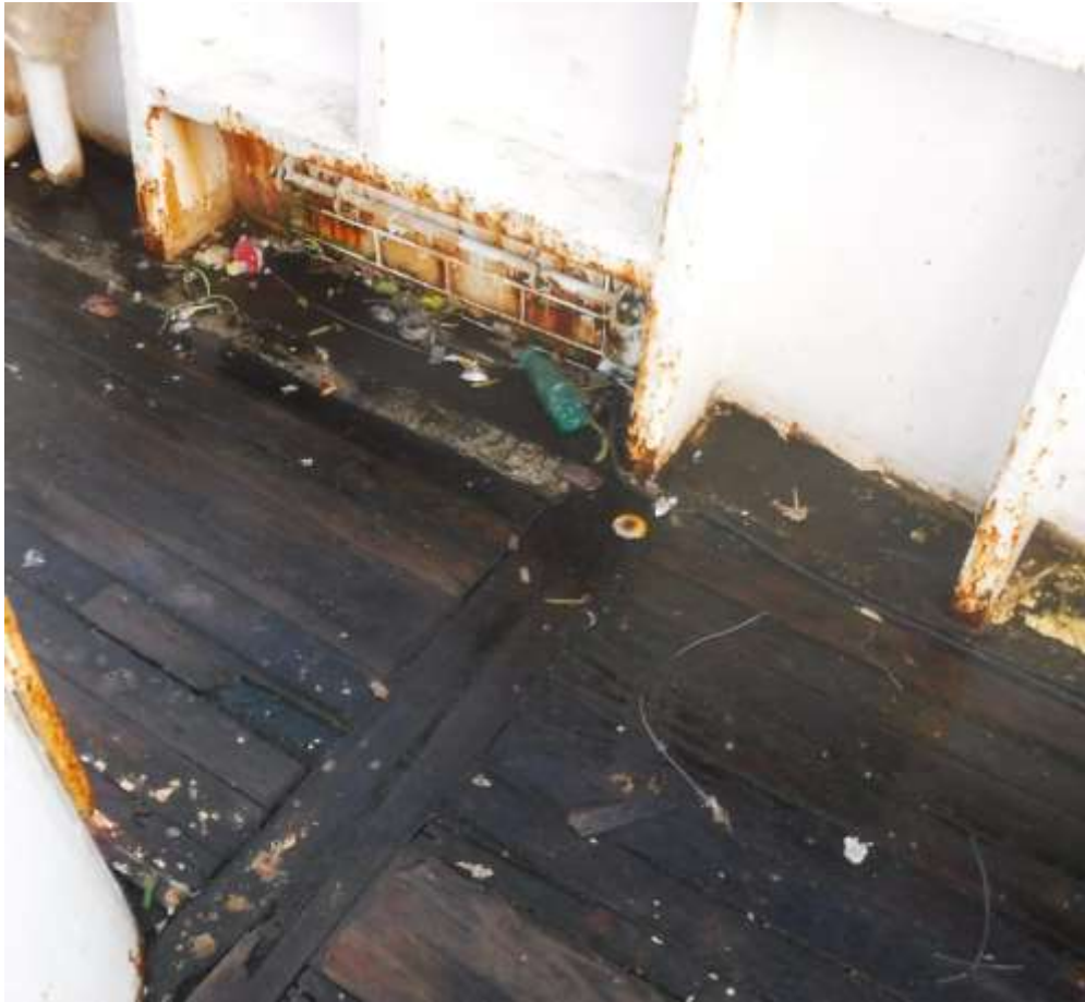
Image 7: Rubbish on a deck in the vicinity of scupper
